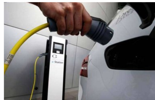
CHARGING POINTS FOR E-CARS
